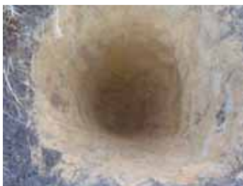
Photograph of test pit showing dry conditions and no evidence of a basin liner
